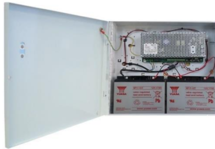
Figure 7 – Battery backup supply
