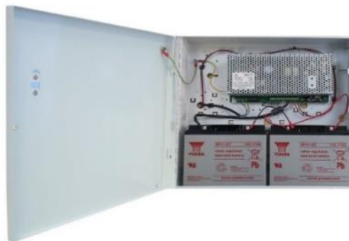
Figure 7 – Battery backup supply
