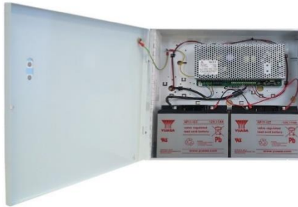
Figure 7 – Battery backup supply
